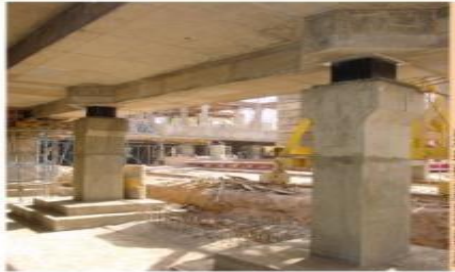
Figure 13 Piers with the lead-rubber bearings at Bhuj District Hospital
