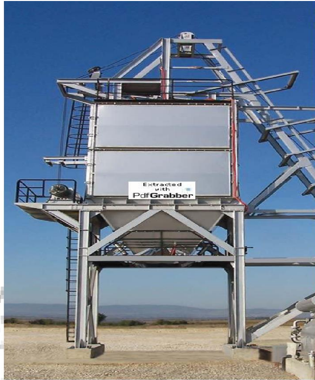
Fig.Hot mix storage silo
