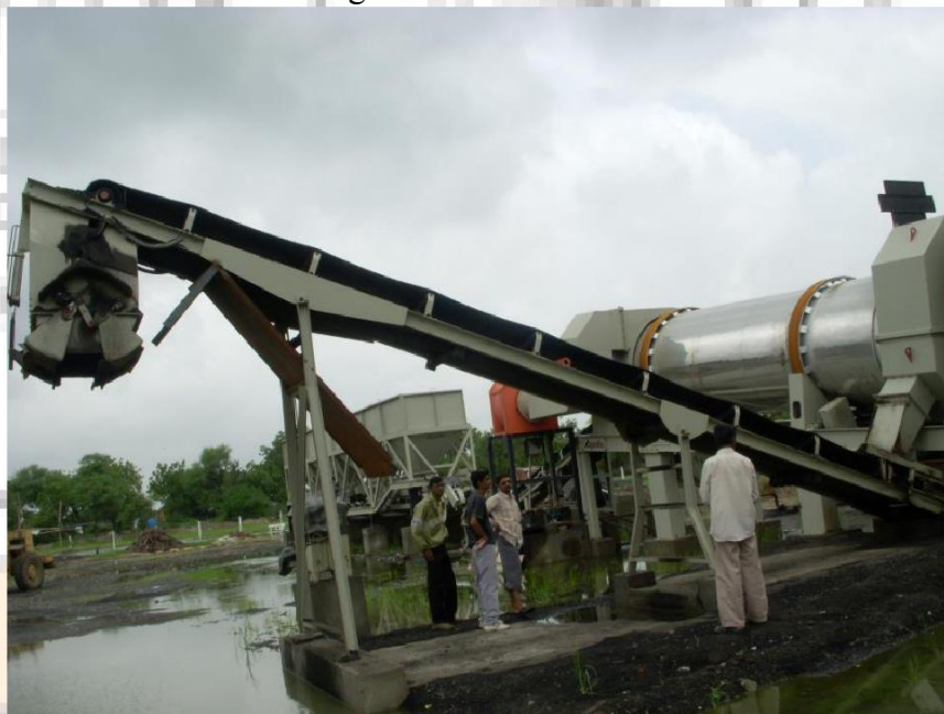
Fig. Load Out Conveyor
