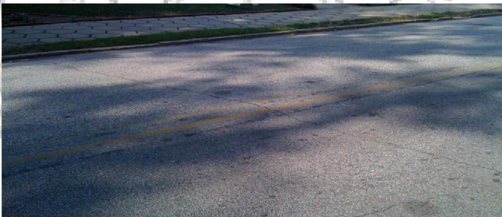
Fig. Transverse Cracking
