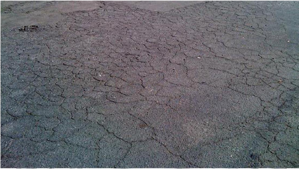
Fig. Alligator Cracking
