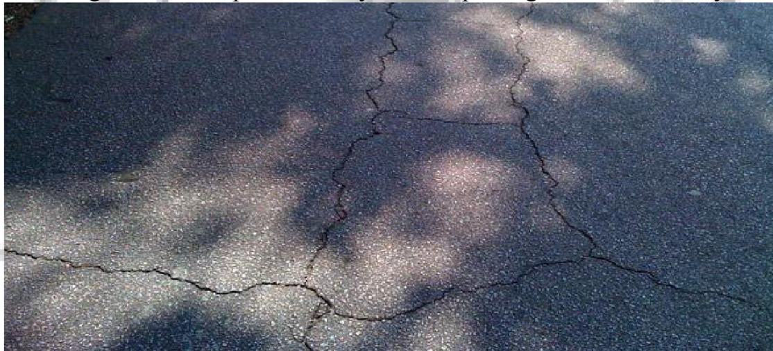
Fig. Block Cracking
