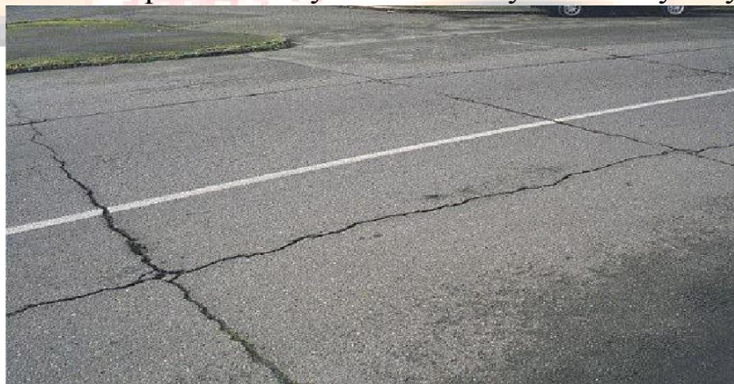
Fig. Joint Reflection Cracks
