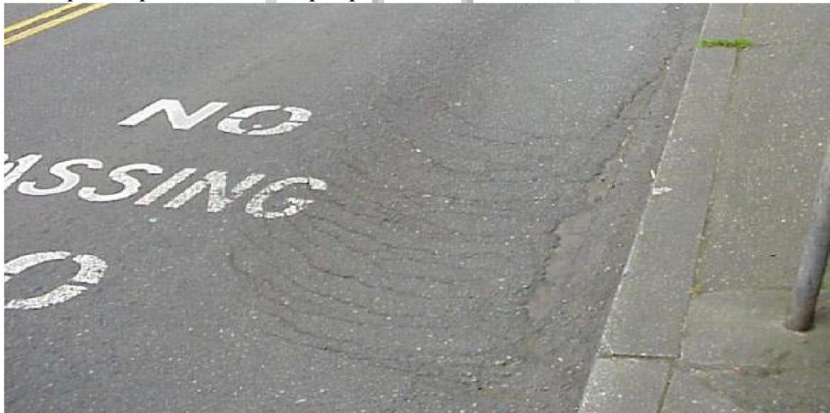
Fig. Slippage Cracks
